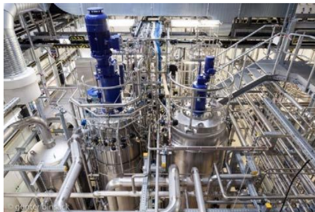
Leuna demo plant
